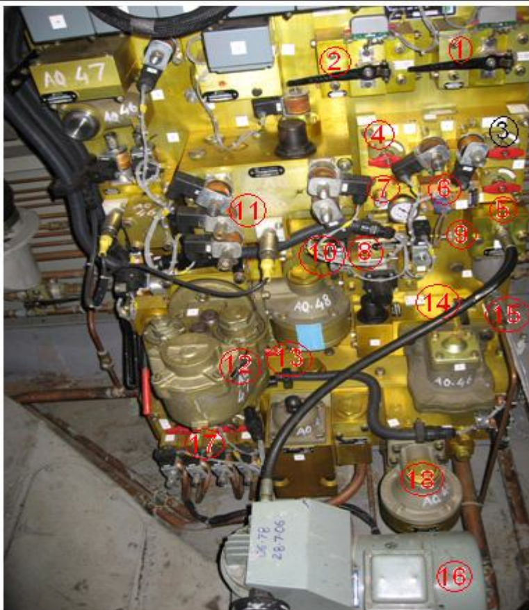
Fig - Pneumatic Panel
